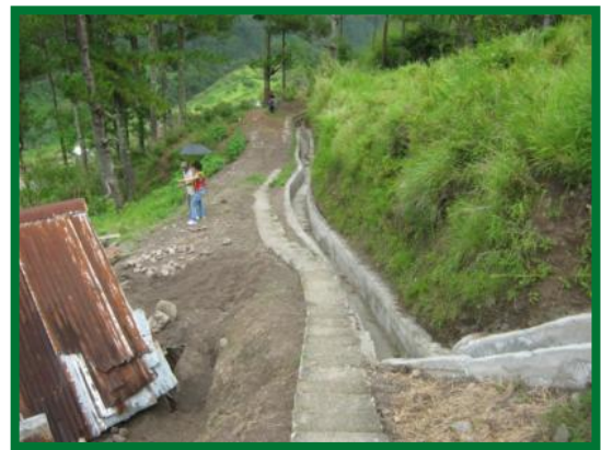
Figure 18 - Example of a small-scale drainage structure that mitigates water flowing onto the road
