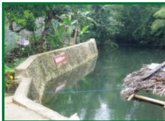
Figure 5 - Example of a river wall or riverbank slope protection used as a flood control structure.
