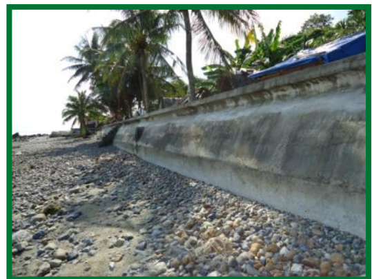
Figure 2 – A seawall structure with a distinctive vertical wall shown at low tide (Camarines Sur)
