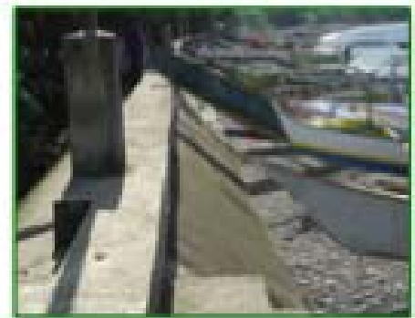
Figure 3 - A revetment structure showing a sloped face shown at low tide (Camarines Sur)
