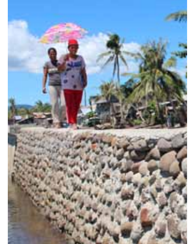
Nelida Balaes and Maricel Velasco proudly show off the sea wall they built themselves through Kalahi-CIDSS which helped keep their village safe from Yolanda
