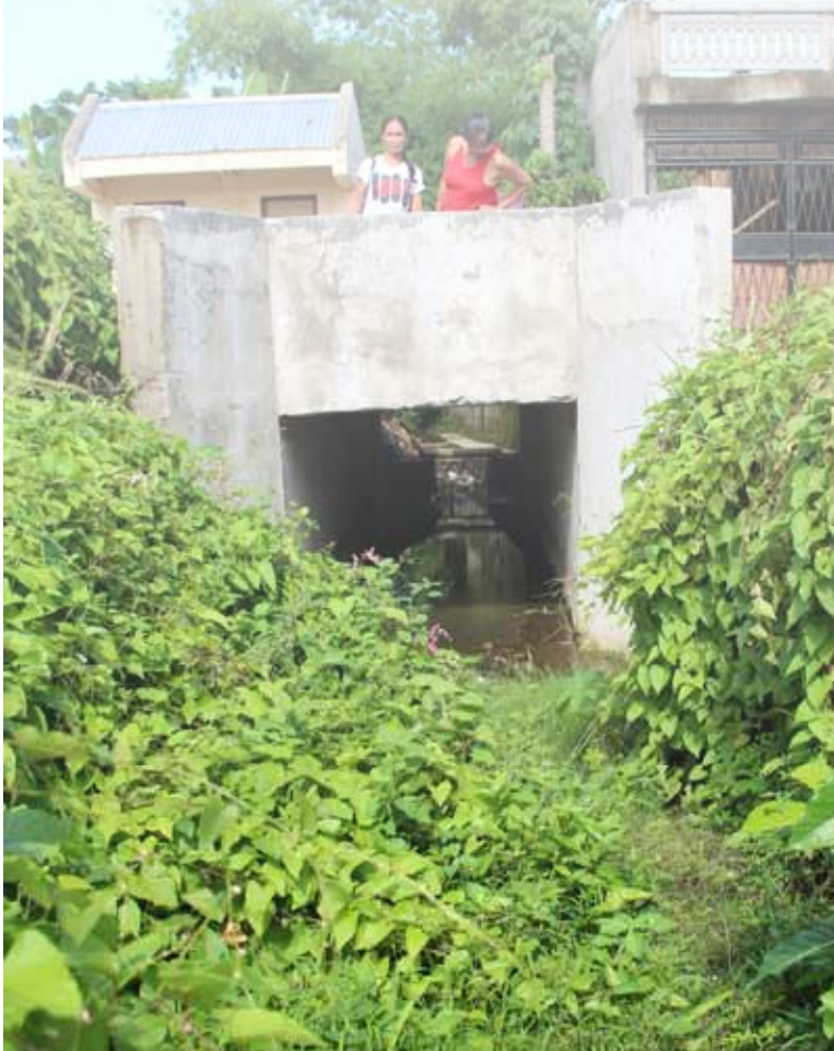
Saving the living and the dead. The community-managed construction of the drainage system in Zone 2, Puro Batia in Libamanan, Camarines Sur now unclogs the stream in the municipal cemetery that had brought flooding during the rainy season to about 70 households who live in the vicinity.
