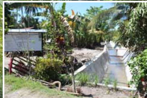
Before and after: Foreground – The construction of the Kalahi-CIDSS slope protection sub-project by the residents; Background – the completed structure
