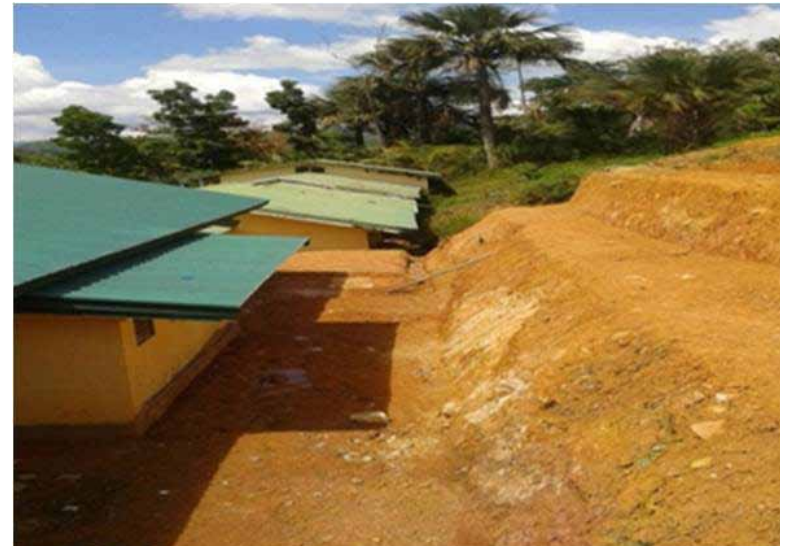
The actual completed 1 unit 2-classroom building of Pangi Elementary School landscaped through Soil Bioengineering Technique with benching and vegetation
