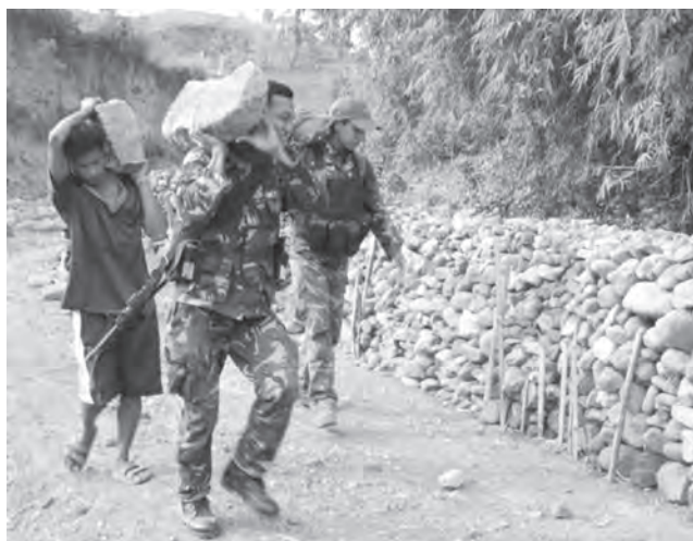
WHILE working at the construction site, soldiers carry both their rifles and sacks of stones to be used in constructing the bridge's approach
