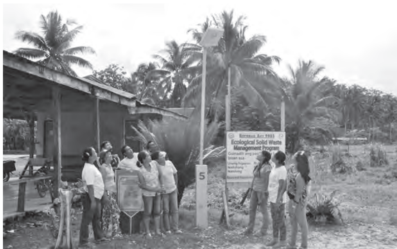
Kalahi-CIDSS volunteers installed their solar streetlights to lessen the incidence of crimes in their community
